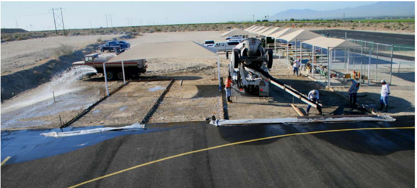
Concrete forms in place and surface being watered in preparation for concrete pour.
